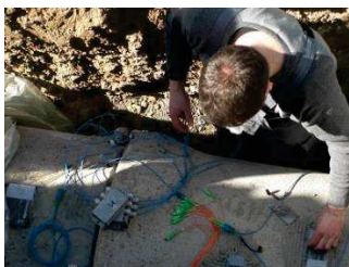
Fig 3 Installation of fibre optic sensors for the SHM of a sewerage tunnel.
